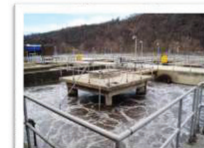
Raw Sewage Plants
